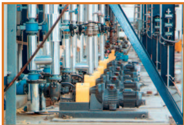
Impianto chimico in Cina Chemical plant in China
